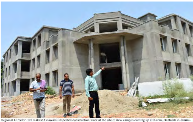
Regional Director Prof Rakesh Goswami inspected construction work at the site of new campus coming up at Keran, Bantialab in Jammu.
