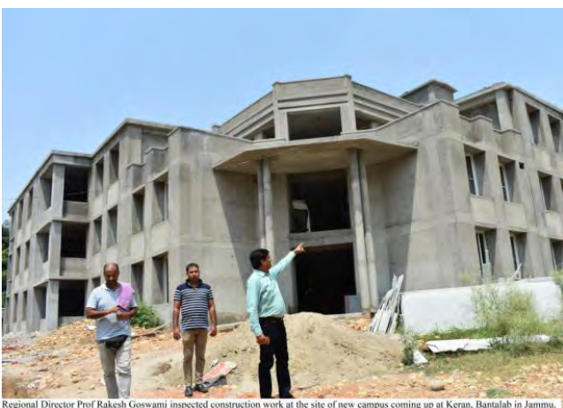
Regional Director Prof Rakesh Goswami inspected construction work at the site of new campus coming up at Keran, Bantalah in Jammu.
